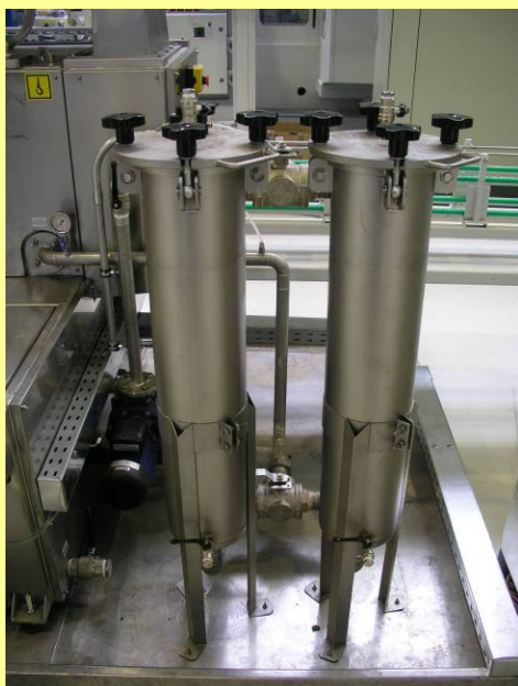
Pic. 3: Double-switch filter as bag filter in the pressure line of the cleaning pump incl. optical/electrical integration in the system control
