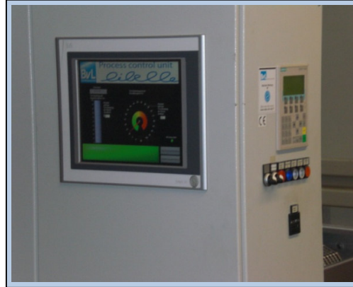
Pic. 2: Indication of the current process status in the control cabinet
